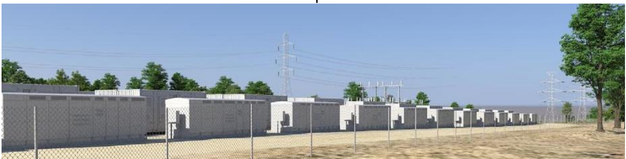
Figure 5 Constructed Battery Storage Facility
